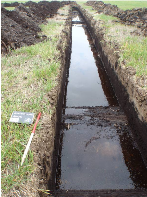
Plate 4 (left) Northwest-southeast arm of the excavation showing peat deposits and complete groundwater encroachment, looking northwest Plate 5 (below). Section 1 with large trunk of “bog oak” at the base. Looking northeast
