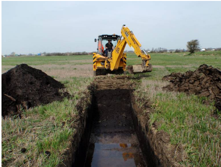
Plate 1. Commencement of excavation showing Queen Elizabeth Way in the distance and the rapid encroachment of groundwater in the trench. Looking approximately northwest
