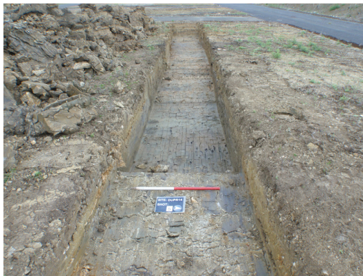
Plate 8. Trench 3 after excavation showing the backfilled cut for mains water at the front of the trench and an electrical service in the centre. Looking west
