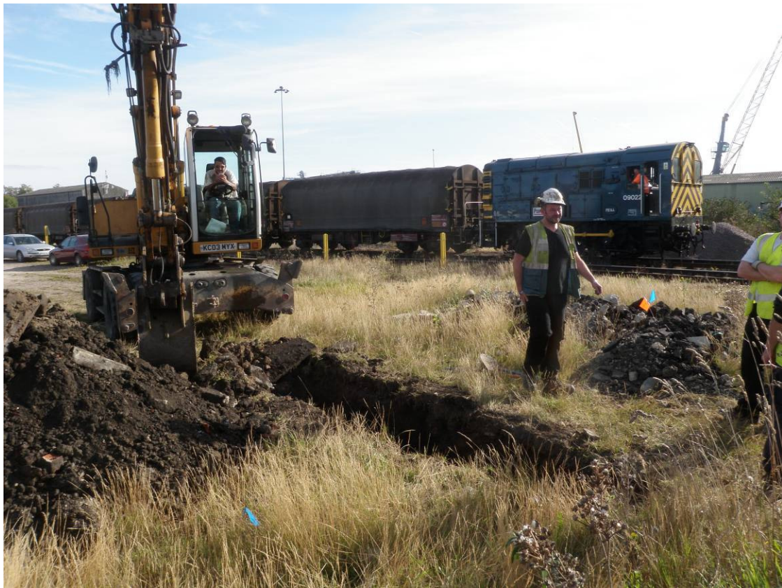
Plate 6. Excavating trial pit 03DRTP04 on line of proposed new road, looking northeast
