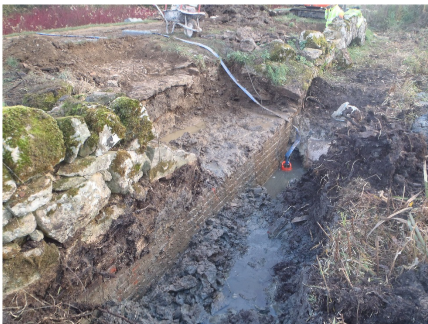
Plate 5 – The investigation area following excavation showing the brick retaining wall (1105) and limestone superstructure (1104), looking southeast
