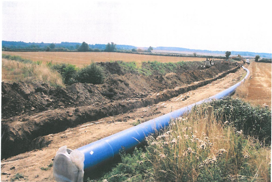
Plate 2 General view showing methodology for pipe trench excavation within field 12B, looking southwest
