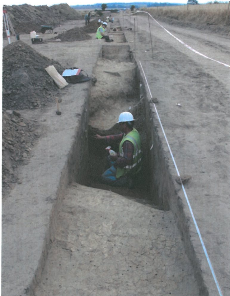
Plate 12 Area 2, general working view along pipe trench, ditches [1041] and [1040] in foreground, looking southwest
