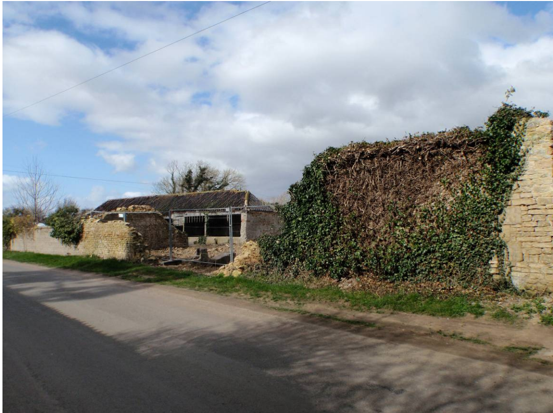
Plate 17 – Building 2 - Collapsed building, south side, looking northwest
