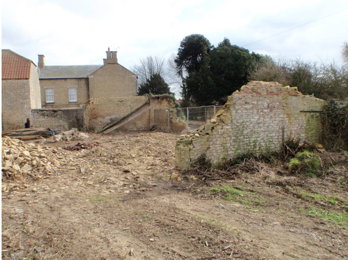
Plate 15 – Building 2 - Collapsed building, general view, looking southeast
