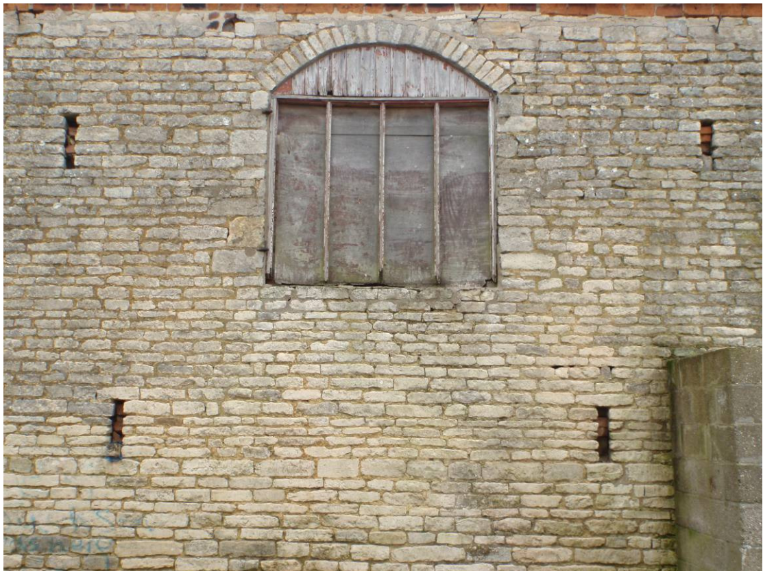
Plate 4 – Building 1 - West side of barn, pitching door and ventilation holes, looking east
