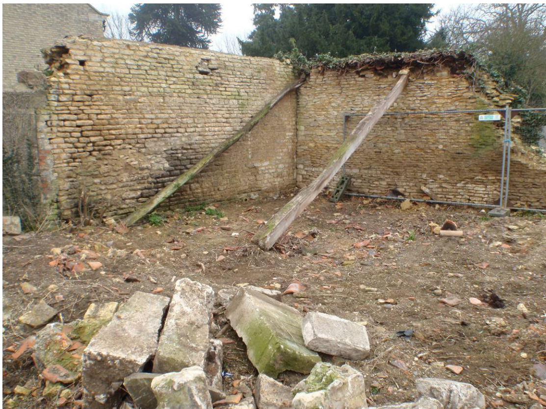
Plate 16 – Building 2 - Interior of collapsed building, eastern end, looking southeast
