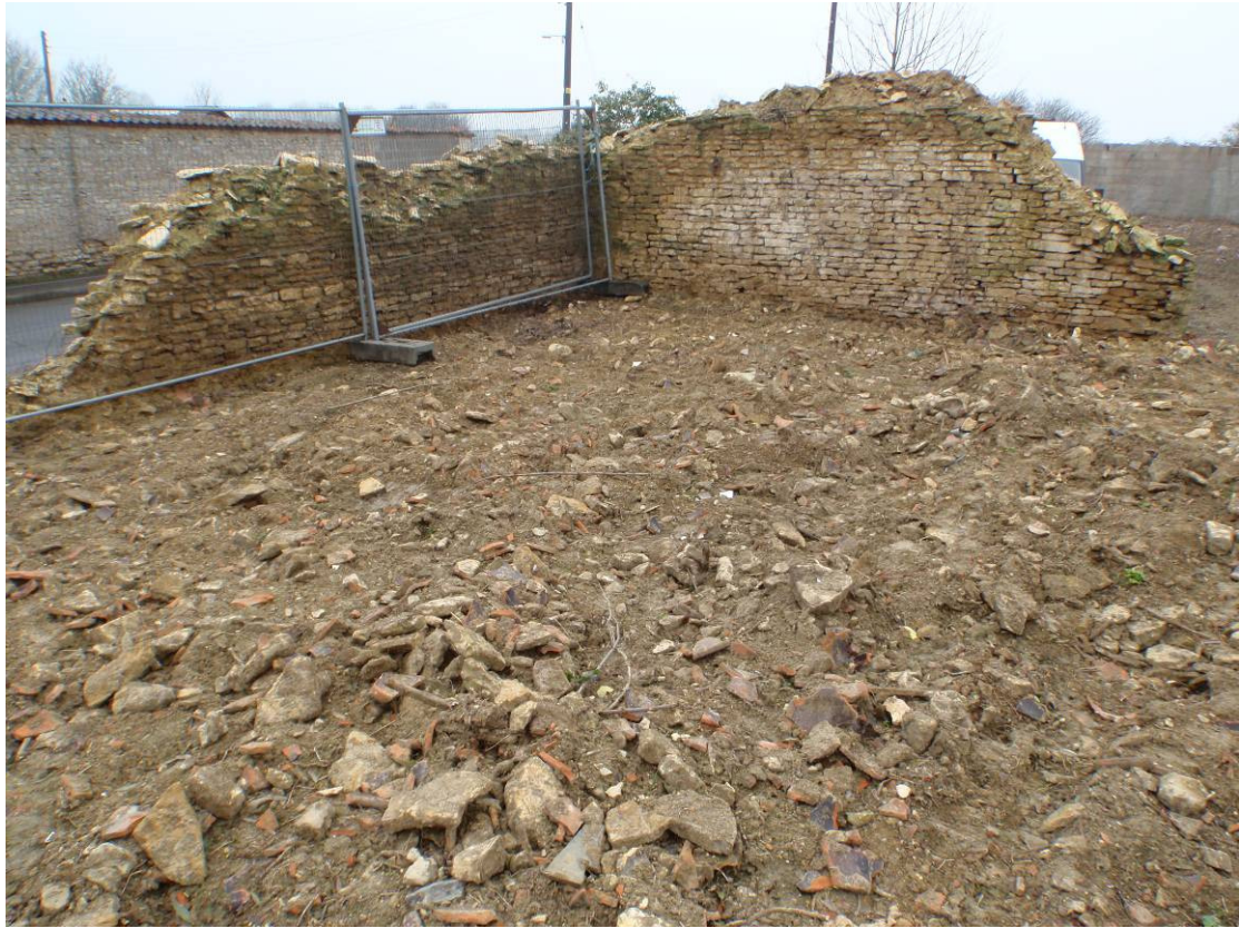
Plate 19 – Building 2 - Interior of collapsed building, western end, looking southwest
