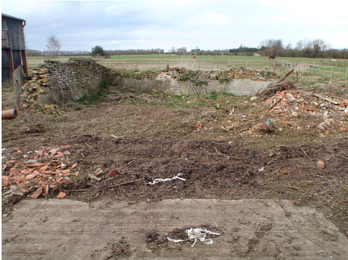
Plate 34 – Other buildings - Collapsed structure north of barn, looking north
