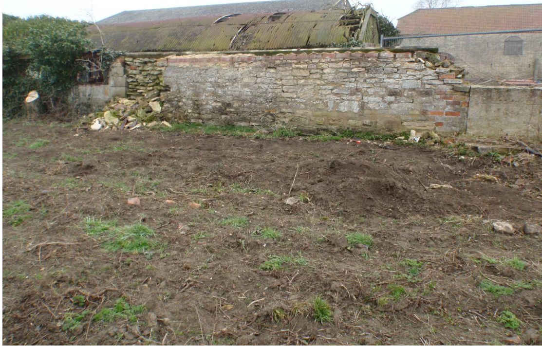
Plate 36 – Other buildings - Stone wall forming part of the western boundary, looking east
