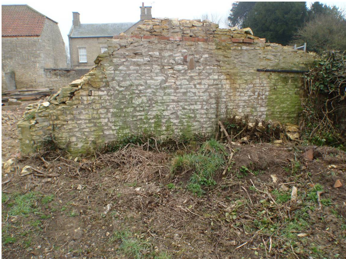
Plate 18 – Building 2 - Collapsed building, west wall, looking east
