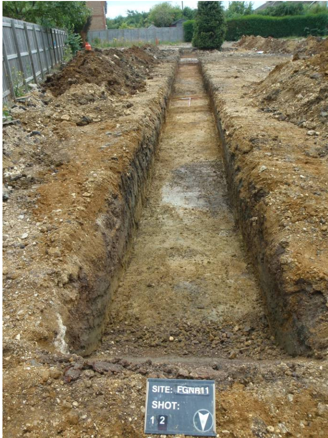
Plate 3. Trench 3 looking south with patch of oil contamination visible
