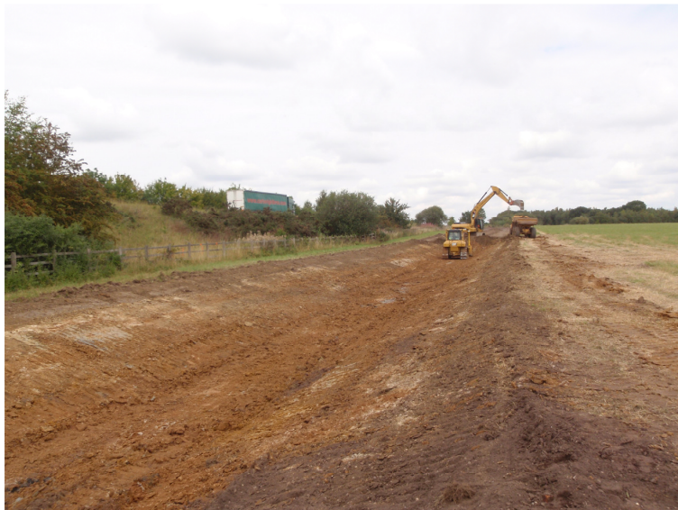
Plate 5 – View showing the new ditch excavation along the southwest boundary of the site, looking northeast
