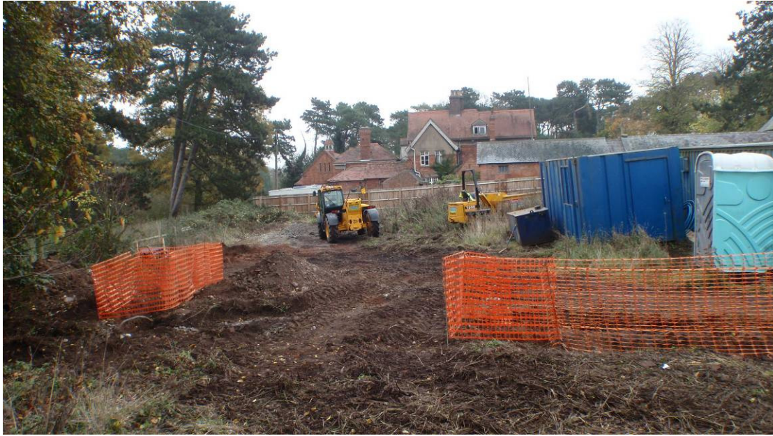
Plate 1. General view of site looking east to Wolvey Hall prior to machining trenches
