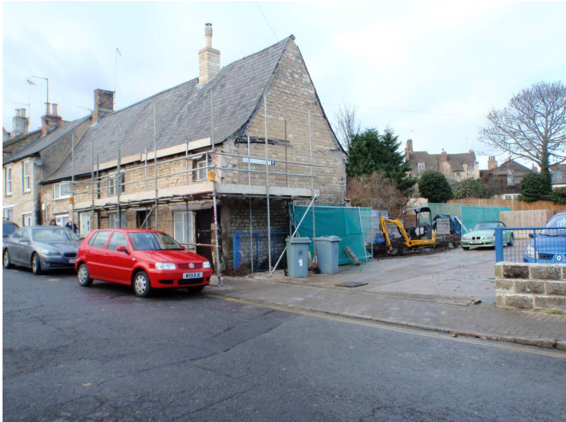
Plate 1. General view of 7 St Leonard's St with work in progress to rear
