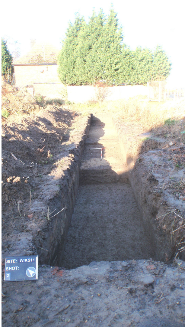
Plate 2 – Trench 1 after excavation, looking northwest (n.b. north arrow pointing in wrong direction)
