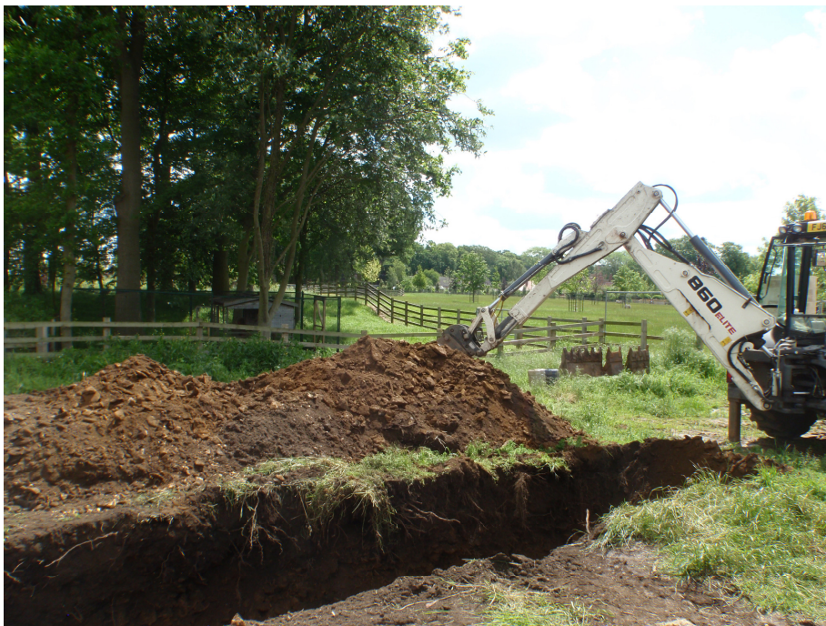
Plate 2 – Machine excavation of Trench 1 with the earthworks in the background, looking southeast
