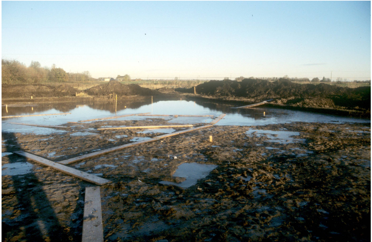
Plate 13. Flooded turbine area looking north, 19 th November 2004
