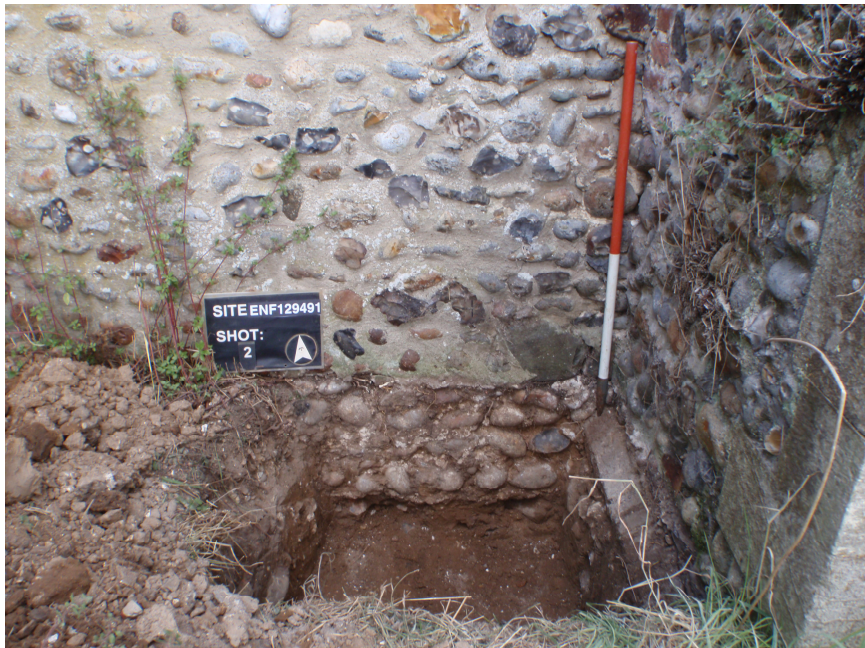
Plate 2 – Test Pit 2, Foundations of the church with buttress overlying earlier buttress (left), looking north
