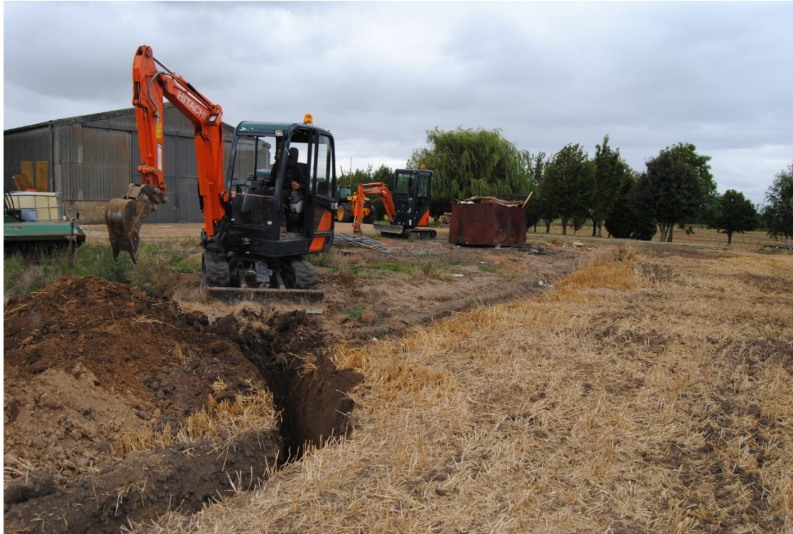
Plate 2 - Looking northwest at the excavation of the cable trench close to the farmyard
