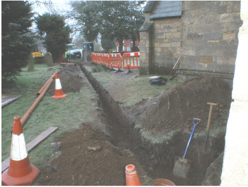
Plate 1 – View showing the extent of drainage works in relation to the church, looking northeast
