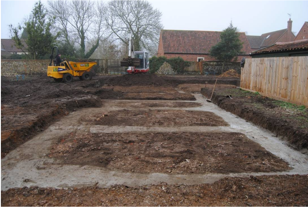
Plate 3. Looking southwest at the eastern part of the building footprint with topsoil removed
