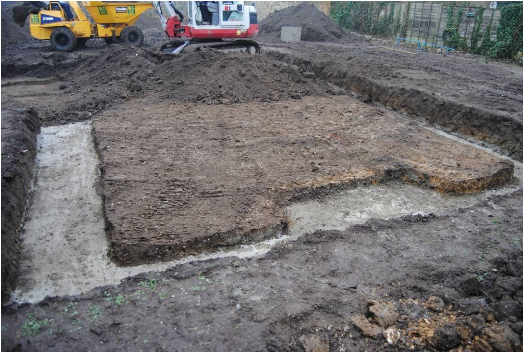
Plate 2. Looking southeast at pit at removal of topsoil within western sections of building footprint.
