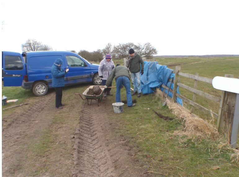
Plate 1 – General view showing the excavation of Pits A and B, looking north
