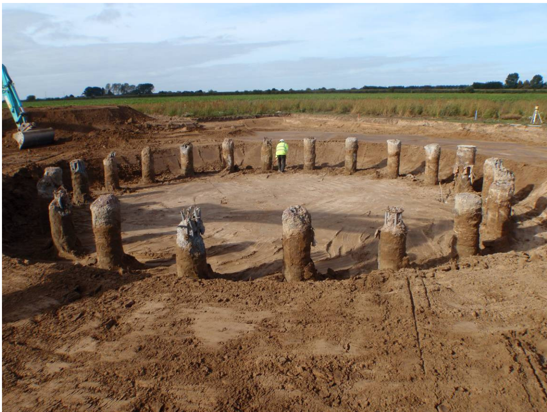
Plate 4. Turbine 3 with concrete piles exposed looking northwest
