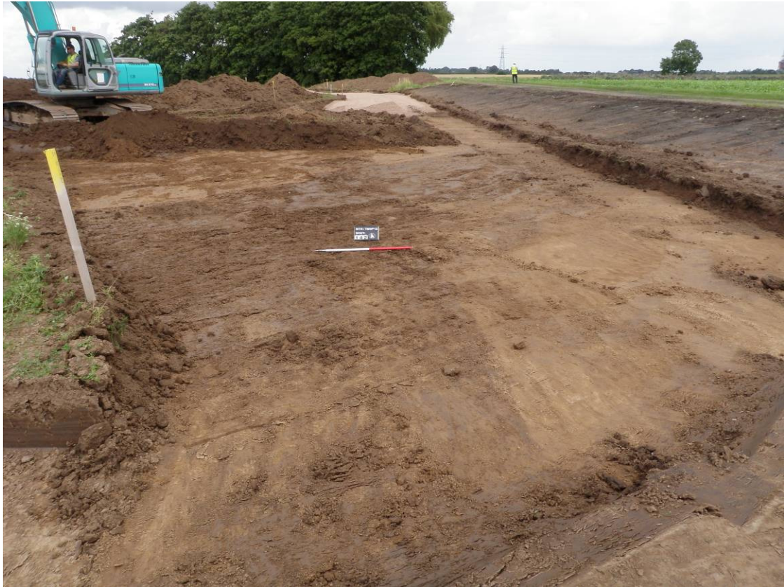
Plate 7. Turbine 5, Ditch [129], parallel to former railway embankment (right), cutting palaeochannel [127], looking north
