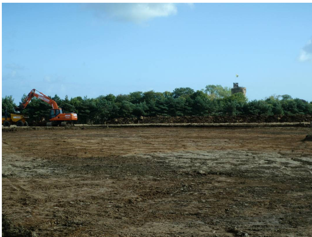
Plate 1. View of the site during topsoil stripping facing south. The castle solar tower in the background.
