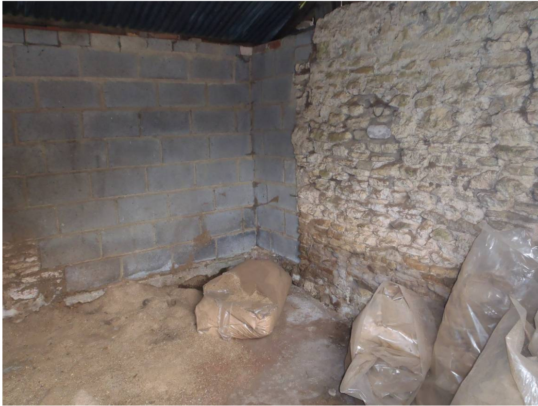
Plate 7 Building 1, southern part, stable compartment at western end showing patching/infill, looking southwest
