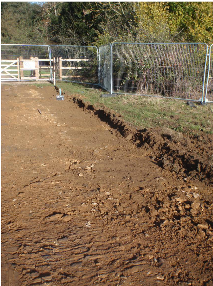
Plate 4 Gully [008], looking north
