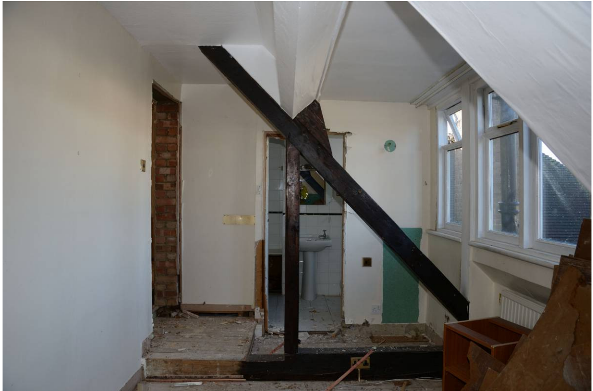
Plate 27. Exposed roof timbers on the northwest side of second floor, looking southwest
