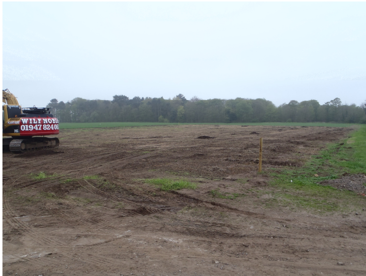
Plate 1. The site prior to the commencement of the removal of the topsoil. Looking approximately southeast
