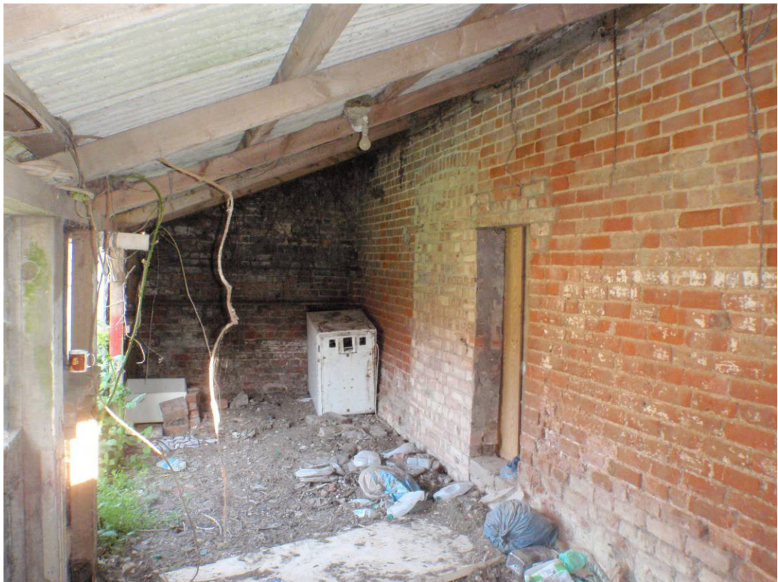
Plate 23: Extension on northeast side of Building 8, showing blocked door and new entry, looking southeast
