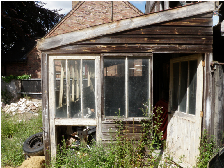
Plate 18. Side view of Building 2, Shed B showing the pitch of the corrugated iron roof
