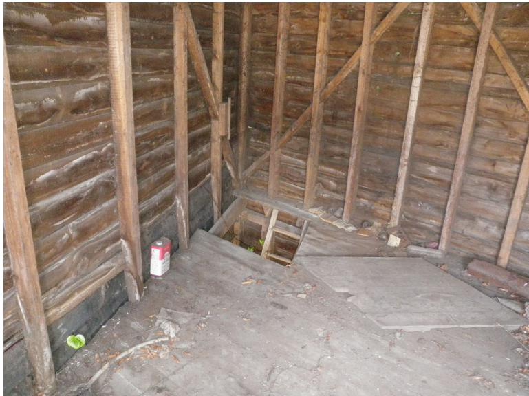
Plate 8. Access to the upper floor of Shed C by means of a hole cut in the floor at the eastern corner of the shed.
