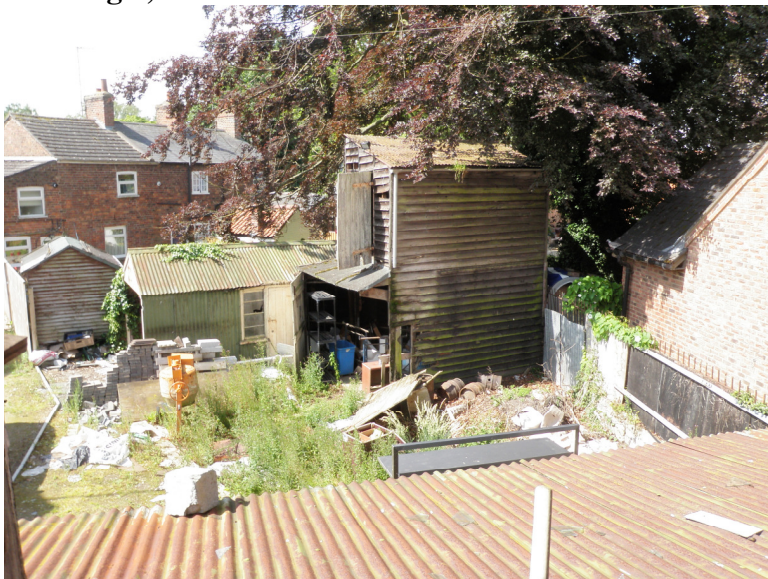
Plate 5. General view of Building 1, Sheds B and C showing the corrugated iron roofs, the corrugated iron northeastern wall of Shed B and the wooden weatherboard of the two storeys of Shed C. Taken from the first floor of Building 2 Shed A.
