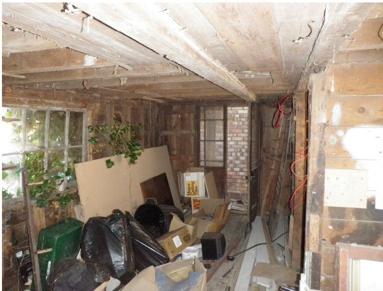
Plate 13. Internal view of the ground floor of Building 2, Shed A. Note the internal dividing wall on the right of the picture and an original doorway at the back left corner.
