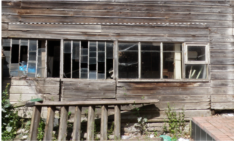
Plate 10. Ground floor windows on the southeast face of Shed A. Note the variations in form and the vertical cuts through the timbers. A long, hinged piece (below the dashed line) that serves no purpose shows re-use of wood from the original form of the structure.
