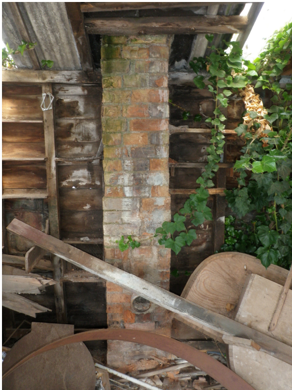
Plate 16 (left). The brick structure with a plastic inlet at the base probably used as a dust extractor. Note the extra light afforded by skylights cut into the roof on either side of the “Chimney”
