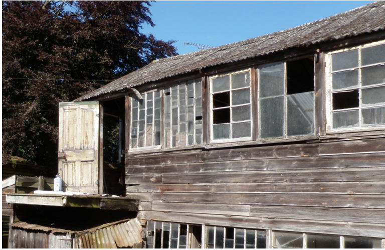
Plate 14. The upper floor of Building 2 Shed A. The access was by a wooden staircase which had since fallen away
