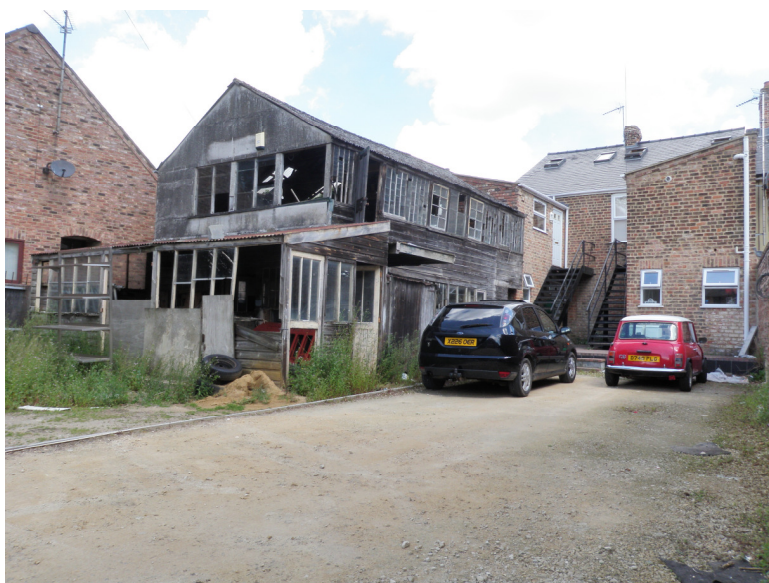
Plate 9. General view of Building 2 showing the buildings fronting onto Market Street at the rear of the photograph.
