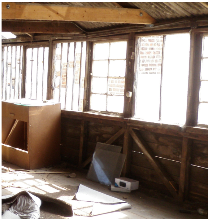
Plate 15. Internal view of the windows and supporting timber structure of the upper floor of Building 2, Shed A
