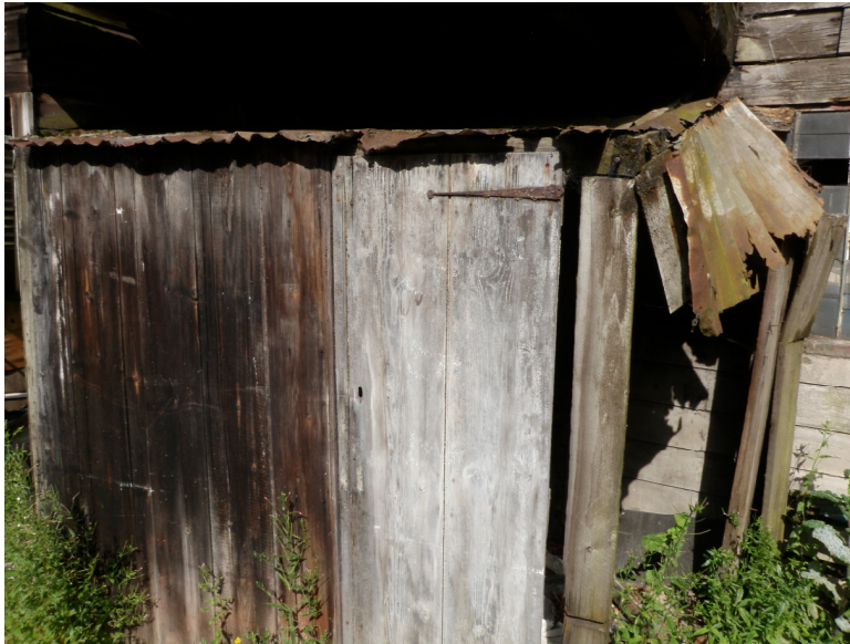
Plate 19. The very basic structure of Shed C. Note the re-use of an old hinged door as part of the outer wall.
