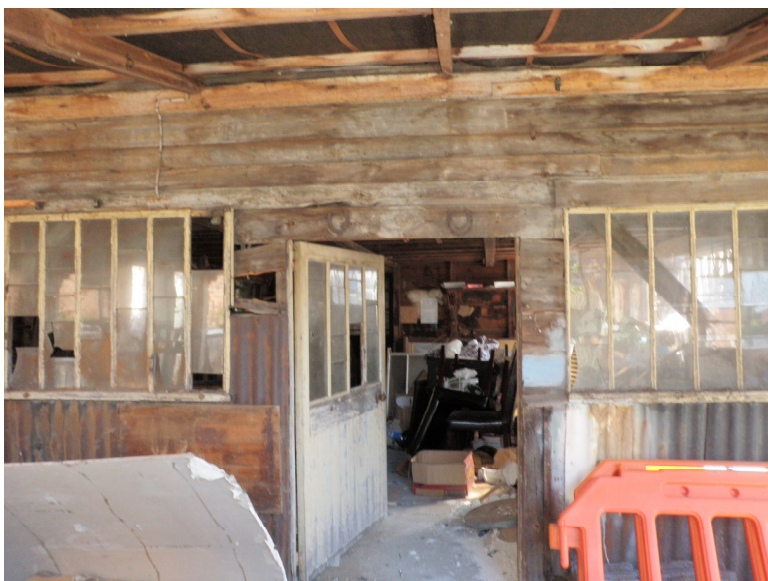
Plate 11. The original exterior wall at the southwest end of Shed A and the original entrance. Note the horseshoes over the doorway and the corrugated iron lower walls.
