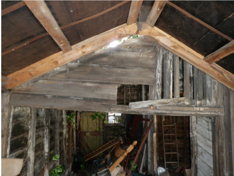
Plate 4. Cut away in southeastern wall from Shed B showing original access door and window
