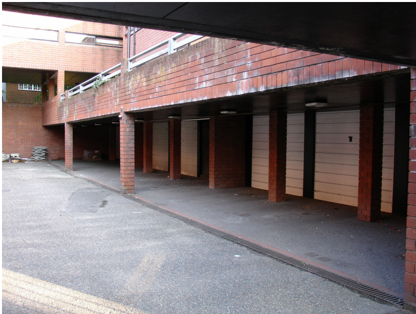
Plate 5 - Another view of the gated yard showing pillars that probably mask stanchions, looking east
