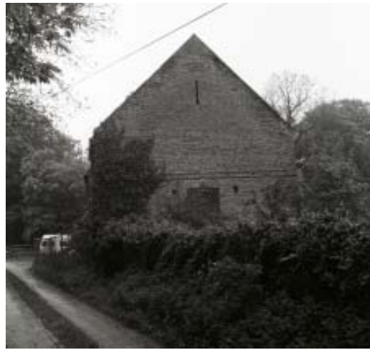
Plate 4 Northern Elevation, showing ventilator window, breather slit, plat-band and sockets, looking south
