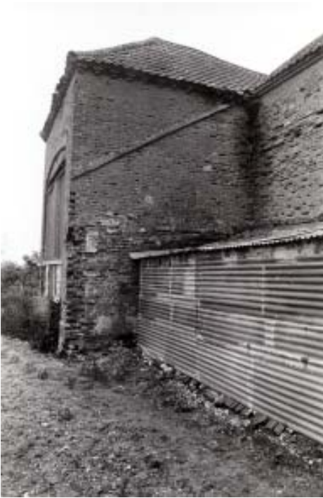
Plate 16 Porch, south side, showing scars of roof lines, looking northeast
