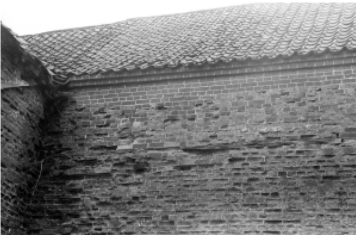
Plate 7 Western Elevation, south side, showing timber lacing and variation in brick, looking east
