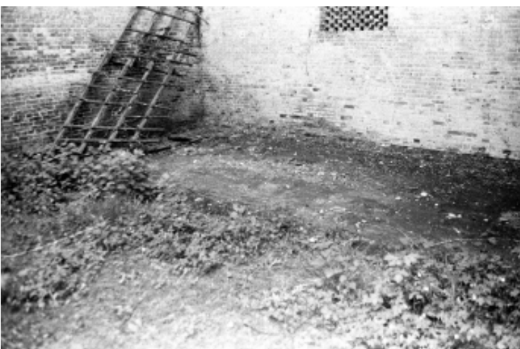
Plate 19 Brick Floor of northern bay, showing damaged/recessed area at northeast corner, looking northeast
