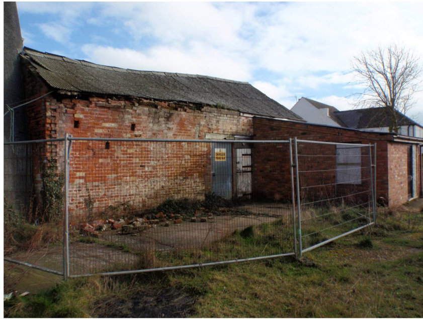
Plate 18. West elevation of the granary showing the modern extension to the southwest corner, the partial wall collapse and the scars at the left that suggest a wall and possible machinery have been removed
