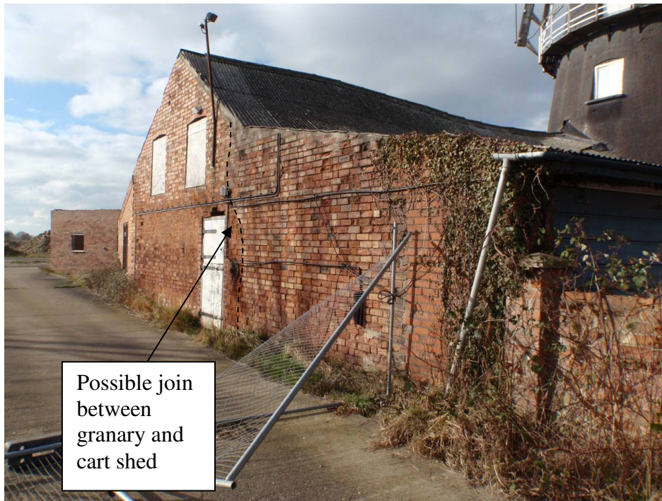
Plate 13. Southern elevation of cart shed showing the different types of brick and bond in the cart shed construction and the possible join between the granary and the cart shed
