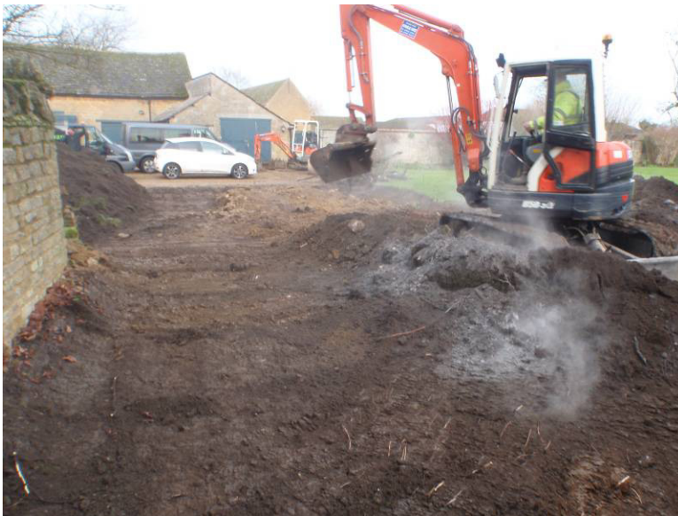
Plate 2. The topsoil stripped from the area where the footings were excavated. Looking northwest
