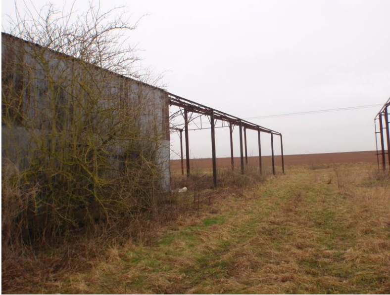
Plate 4. The frame of the second barn from the west showing the additional struts for the mono-pitched roof (removed). Looking northwest
