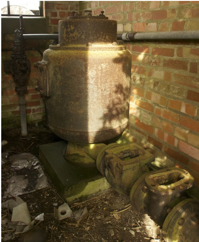
Plate 20. Detail of a boiler, probably located adjacent to the “retting tanks”. The heated water would have been pumped from here to the tanks.
