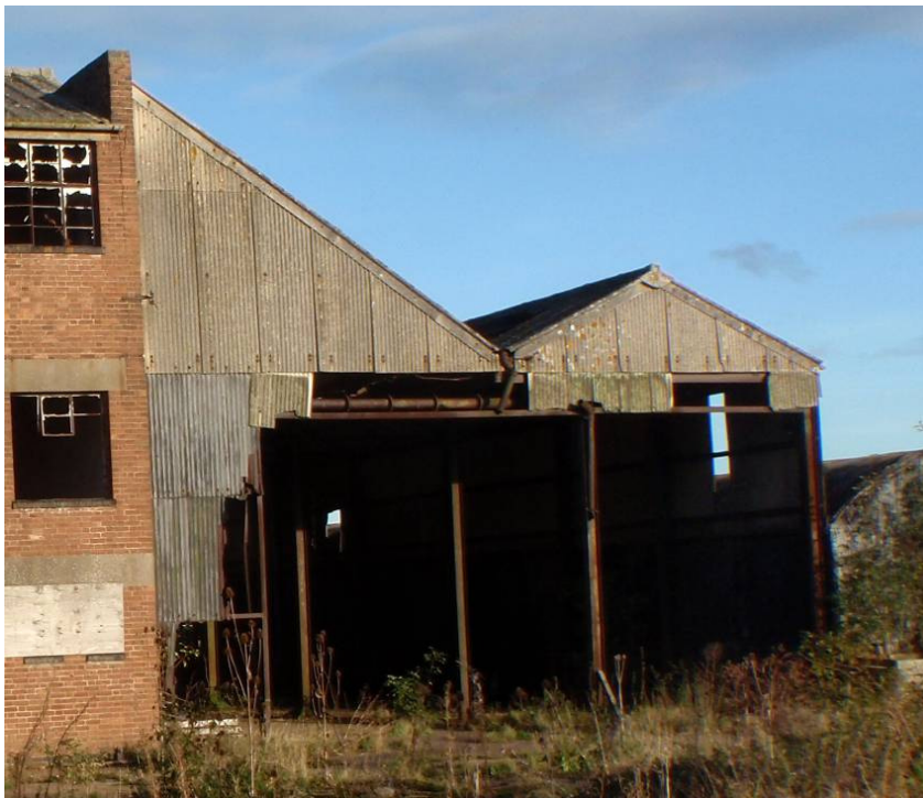
Plate 7. The lean-to steel framed corrugated iron sheds at the southern elevation of the main factory complex. Looking east
