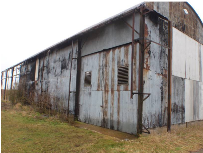
Plate 3. The second barn from the east, entirely enclosed and accessed from the southwest corner. Looking northeast
