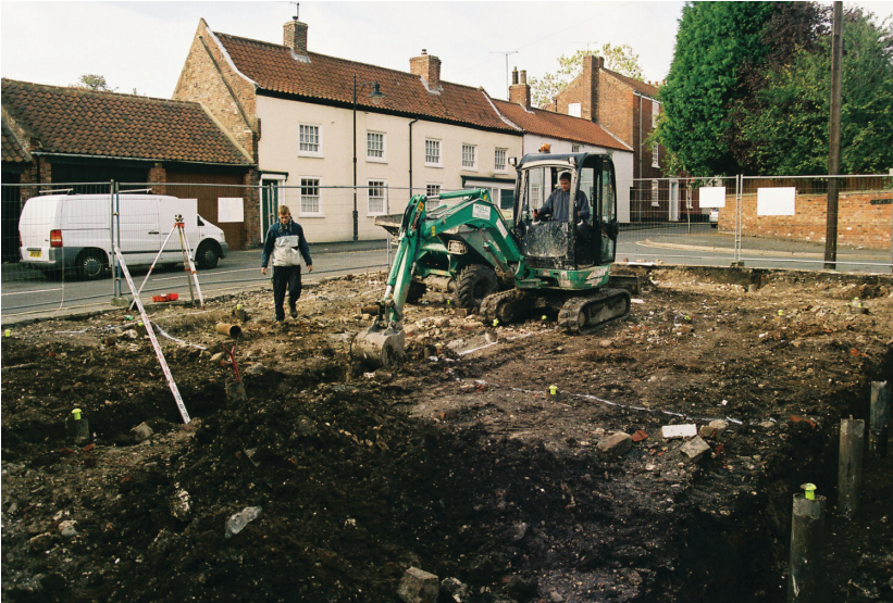
Plate 1 - View across the development area during initial stripping of the site, looking southwest
