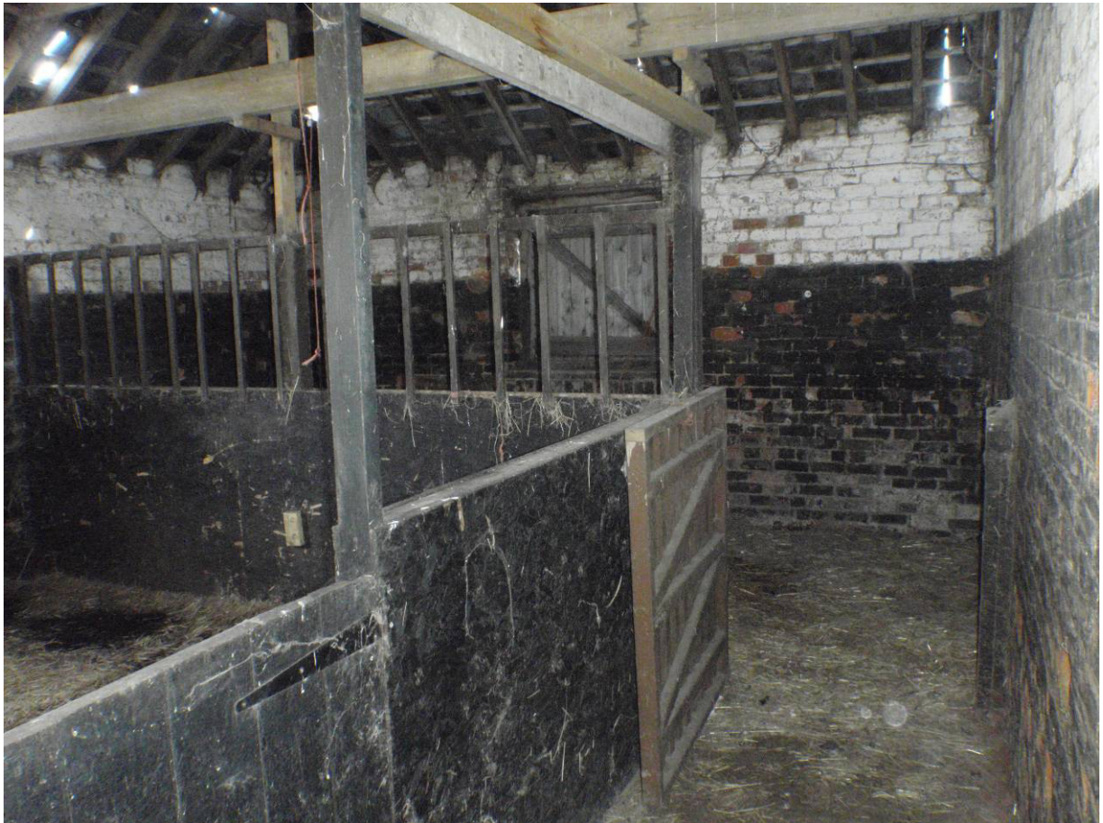
Plate 23. North range, passageway and Room 5 beyond, with Room 4 on left, looking east
