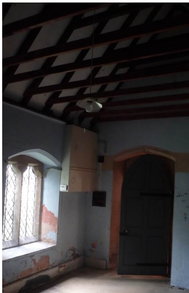
Plate 12 (left). The vestry looking towards the church showing exposed roof timbers and stone arched window
