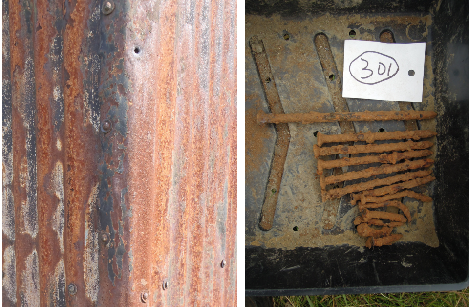
Plate 2 (left). A detail of the nails with washers that attach the corrugated outer to the building's timber frame as seen on an example removed from Belton Park and re-sited at Fishtoft.
