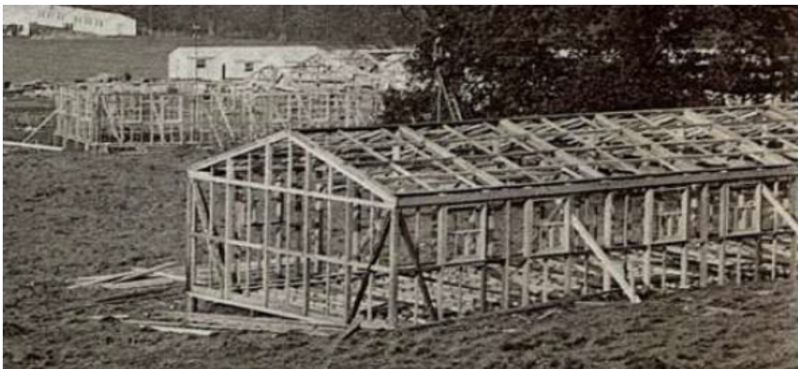
Plate 1. A view of the wooden huts under construction showing the lightness of their frame. Note that where built on uneven ground they have been made level using wooden posts ( image courtesy of the National Trust/Belton House)
