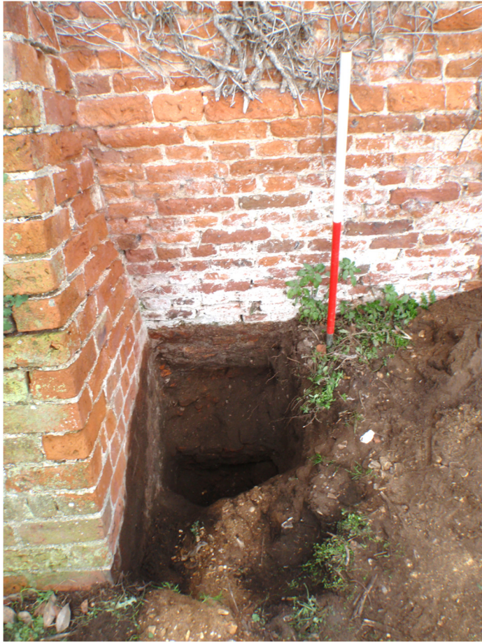
Plate 3. Test Pit 1, Section 1, looking north
