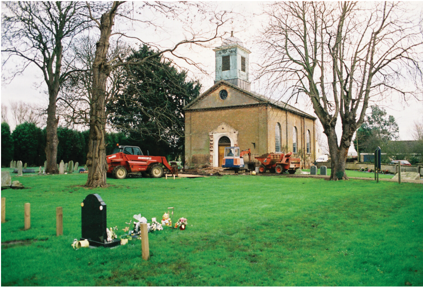
Plate 1 - View of St John the Baptist church following demolition of the west porch, looking northeast
