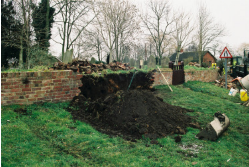
Plate 1 - View of the churchyard wall showing the repairs in progress, looking northeast
