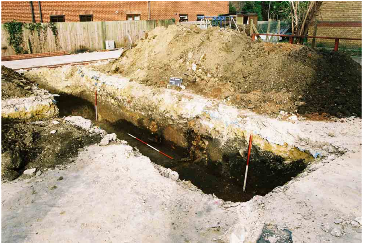
Plate 3 Trench 1, Section 2, showing brick structure (126) etc, and sequence of deposits, looking north
