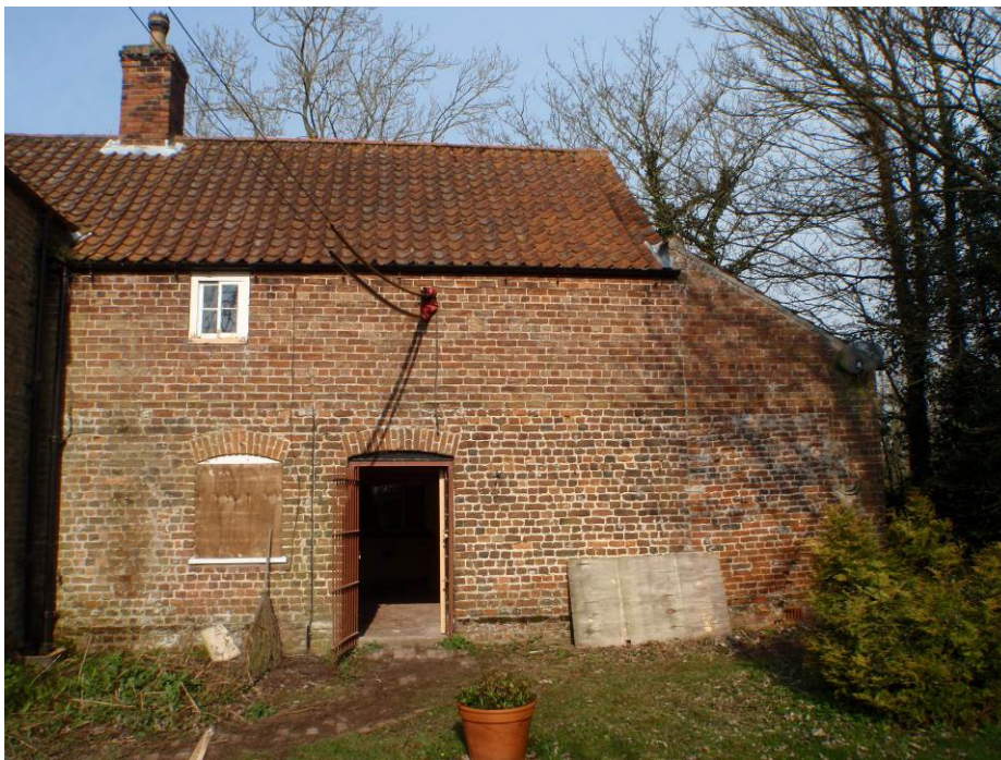
Plate 6. The east elevation of the North-South Range showing four of the probable five phases of construction.
