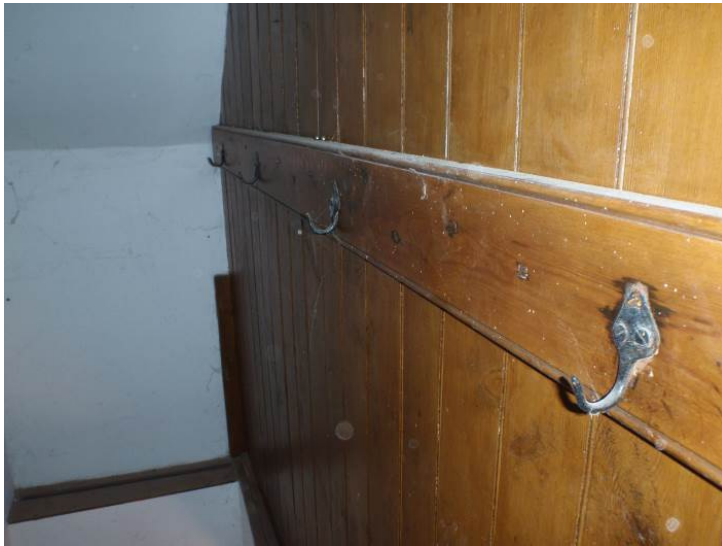
Plate 42. Detail of the metal hooks on the wooden panelling of the 'back stairs' possibly for servant's bells
