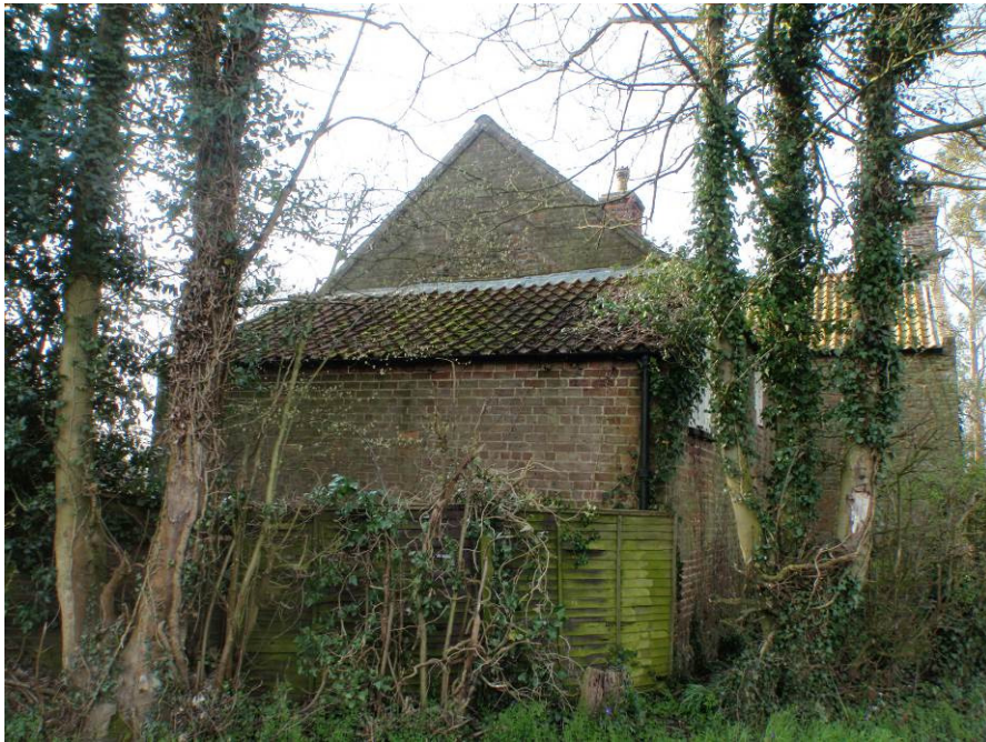
Plate 9. A general view of the north elevation showing the extension and the original gable end of the North-South Range
