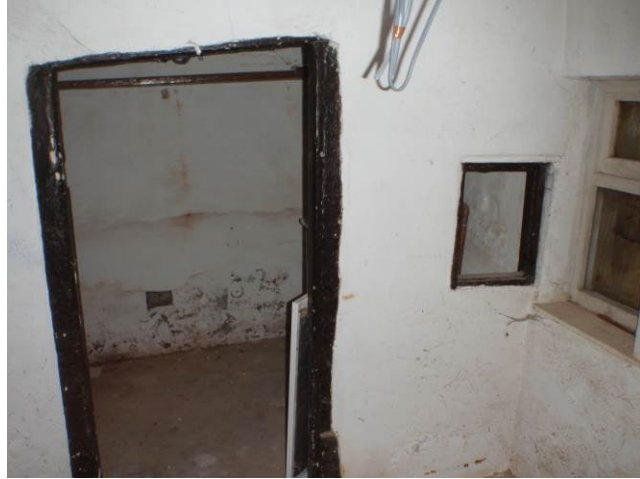
Plate 28 (below). The uneven doorway and hatch to the boiler room to the west and the 20 th century window in the original 19 th century aperture
