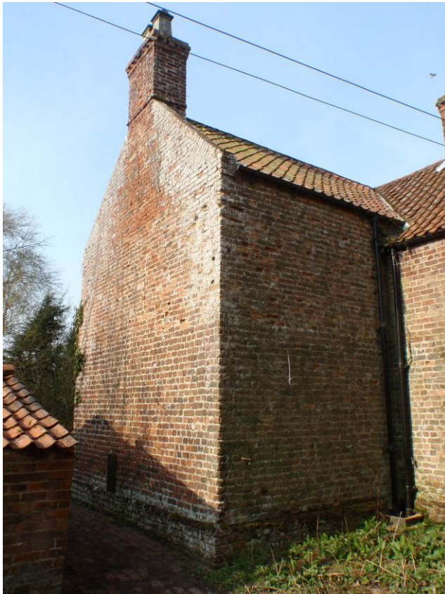
Plate 4 (left). The east elevation and the north elevation of the East-West Range. The east elevation has two triangular 'tumbled' sections at eaves level with associated 'kneelers' in the north elevation
