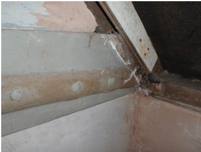
Plate 39. Detail of the iron bracers trip on the tie beam. It is twisted to fold over the wall plate on the west wall
