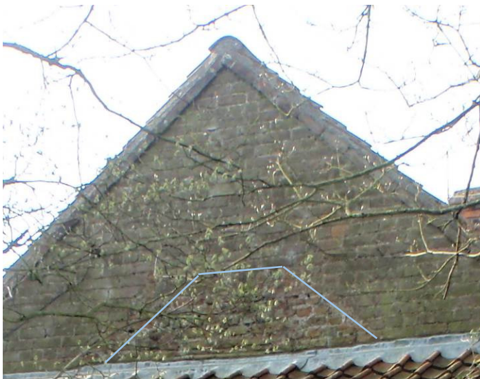
Plate 10. A detail of the north gable end of the North-South Range. The trapezoidal brick infill is highlighted
