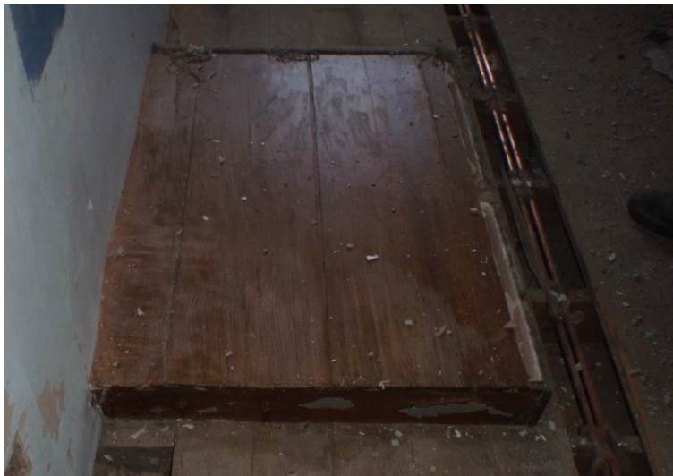
Plate 45. The blocked hatch in Room 10 leading to the Pantry Area below
