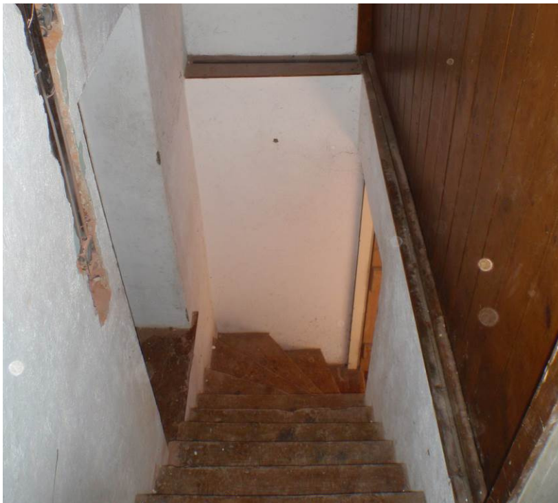
Plate 41. The Back Stairs leading to the mezzanine Room 10 on the left of the picture and Room 3 at the foot of the stairs
