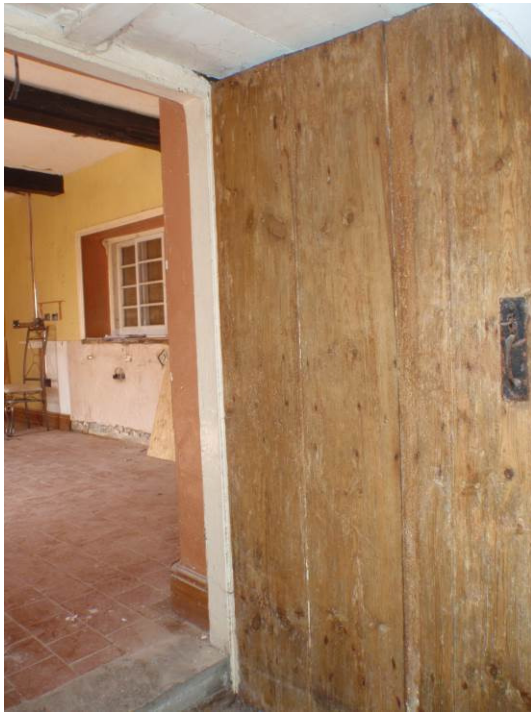
Plate 27 (left). The late 18 th or early 19 th century door from Room 3 to the Pantry Area
