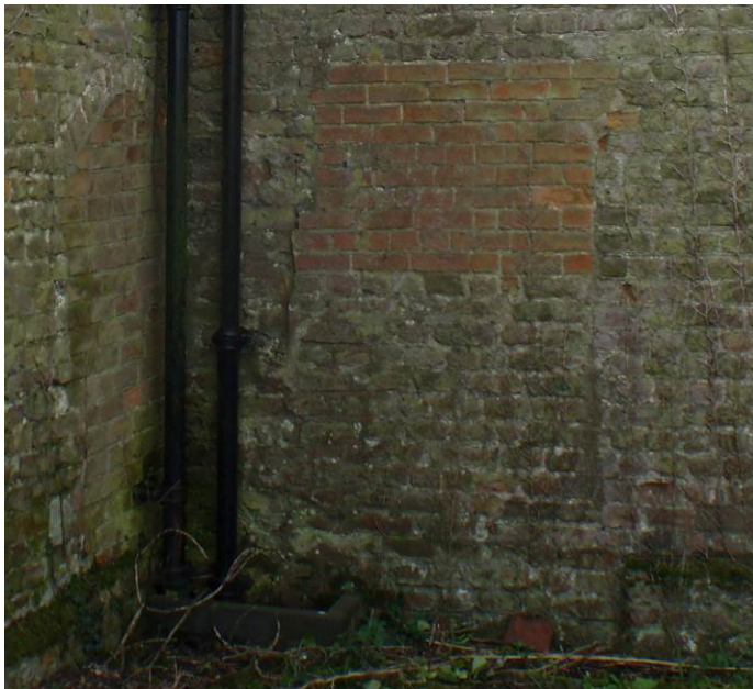
Plate 12 (left). Detail of the dome topped oven feature in the west elevation linking with the blocked opening that was infilled in two phases in the adjacent north elevation
