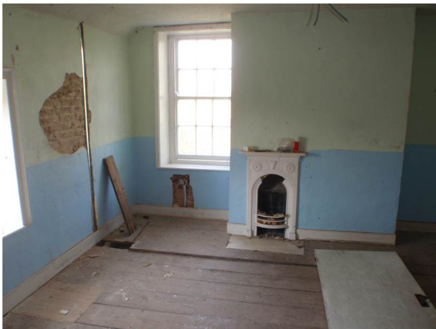
Plate 31. Room 4 with the offset fireplace and the 19 th century surround. The hearth is supported from below in Room 1
