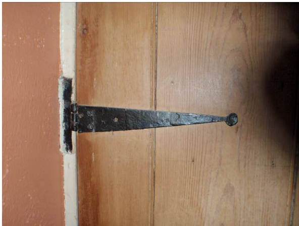
Plate 25. Detail of door hinge on the under stairs cupboard in Room 3, possibly an early hinge on a later door
