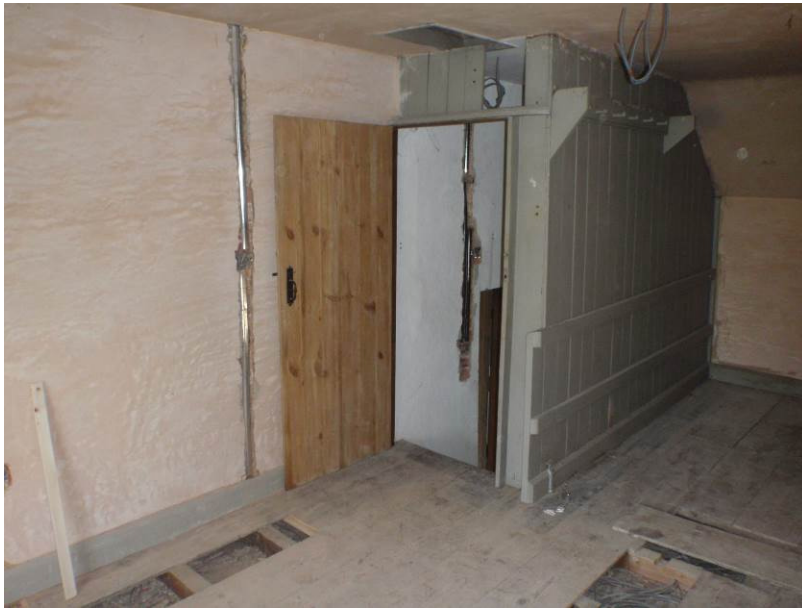
Plate 40. The northeast corner of Room 9 with the wooden surround for the back stairs. The row of coat pegs suggests this was used as separate living quarters
