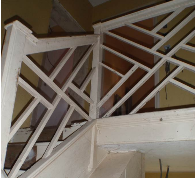
Plate 30. The decorative balustrade panels in the Art Deco style on the Front Stairs
