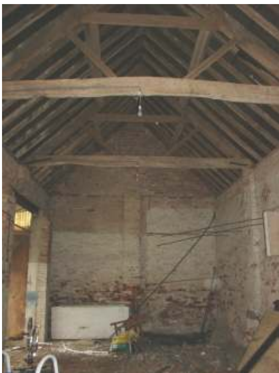
Plate 12 - View of the interior of the barn showing the collar and tie beam truss roof, looking east
