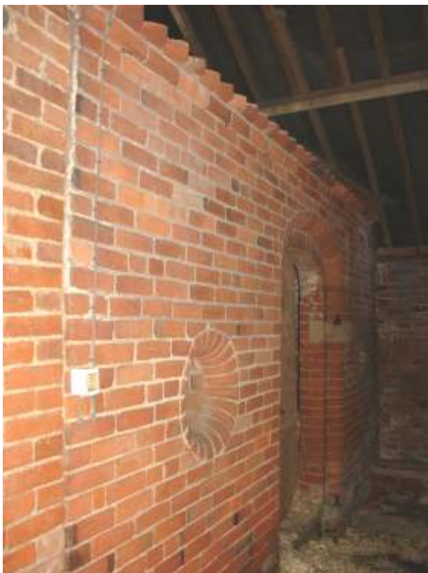
Plate 5 - View of the north range at the eastern end showing decorative brickwork and straight join to barn
