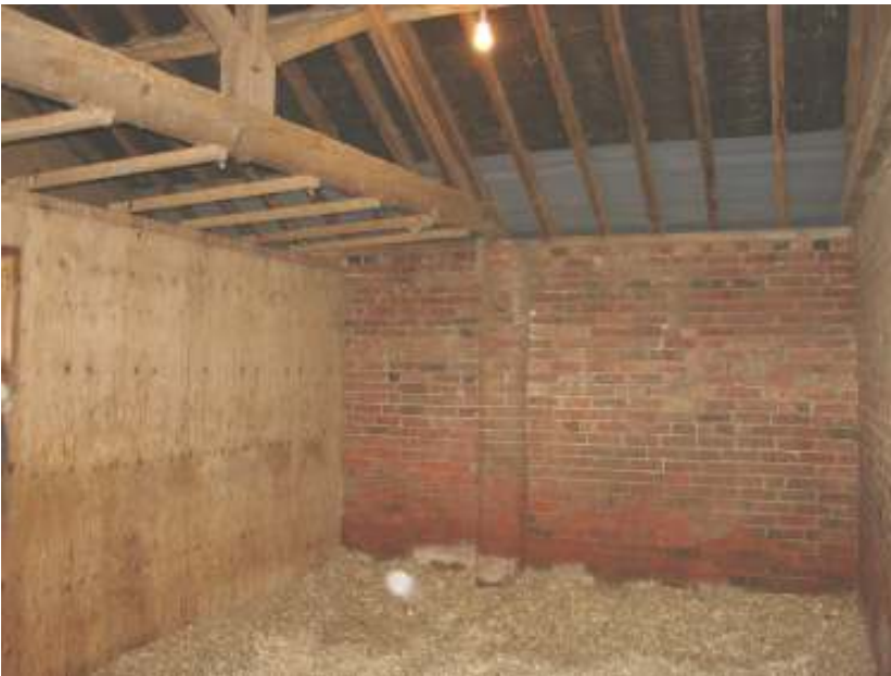
Plate 20 - Interior view of the former cart shed showing internal buttress and recent wooden partitions
