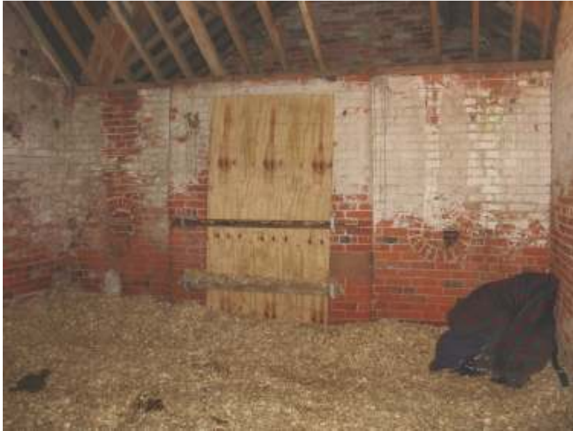
Plate 16 - View of the interior of the east room of the north range, showing the circular brick recesses
