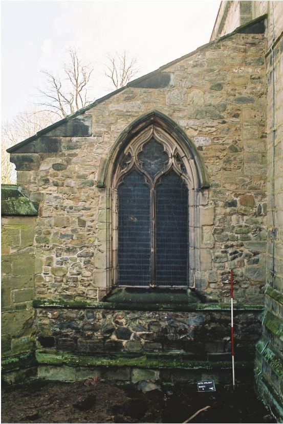
Plate 4 - West facing elevation of the north aisle, prior to excavation, looking east
