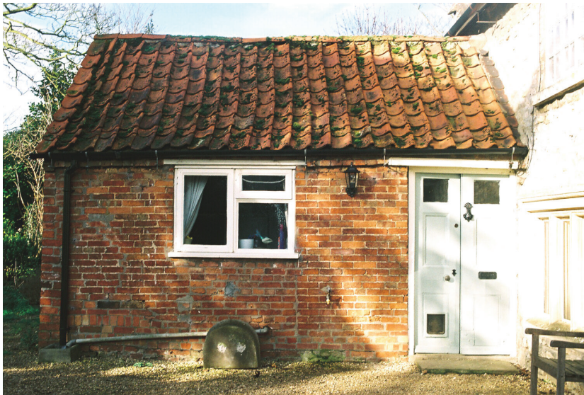
Plate 4 - The east facing elevation showing modern patching to left of picture and ragged joins below the window, looking west
