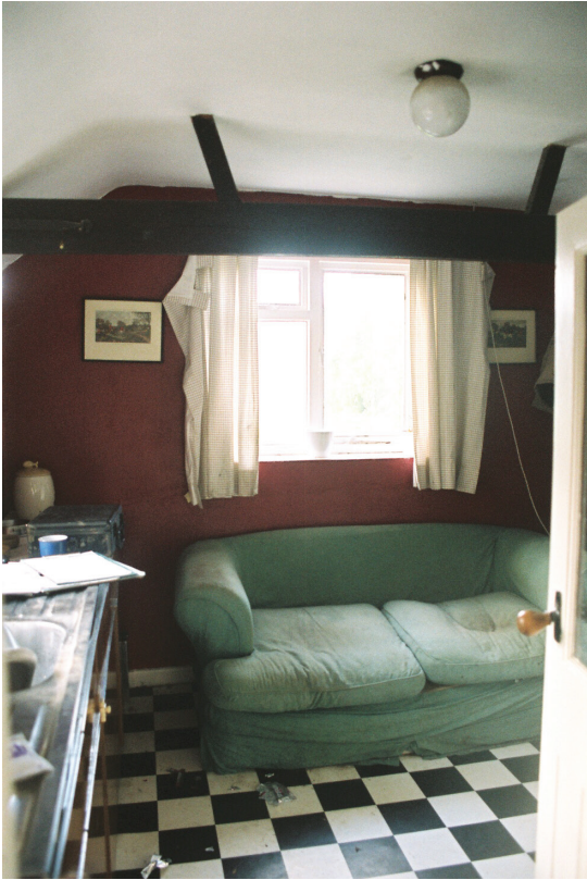
Plate 7 - View showing the larger room within the extension with exposed tie-beams and raking struts, looking south
