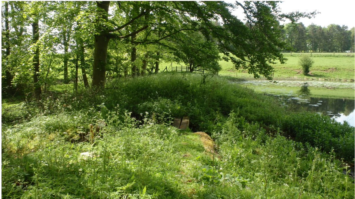
Plate 6 – View of dam, looking south, showing breach and previous concrete repair work
