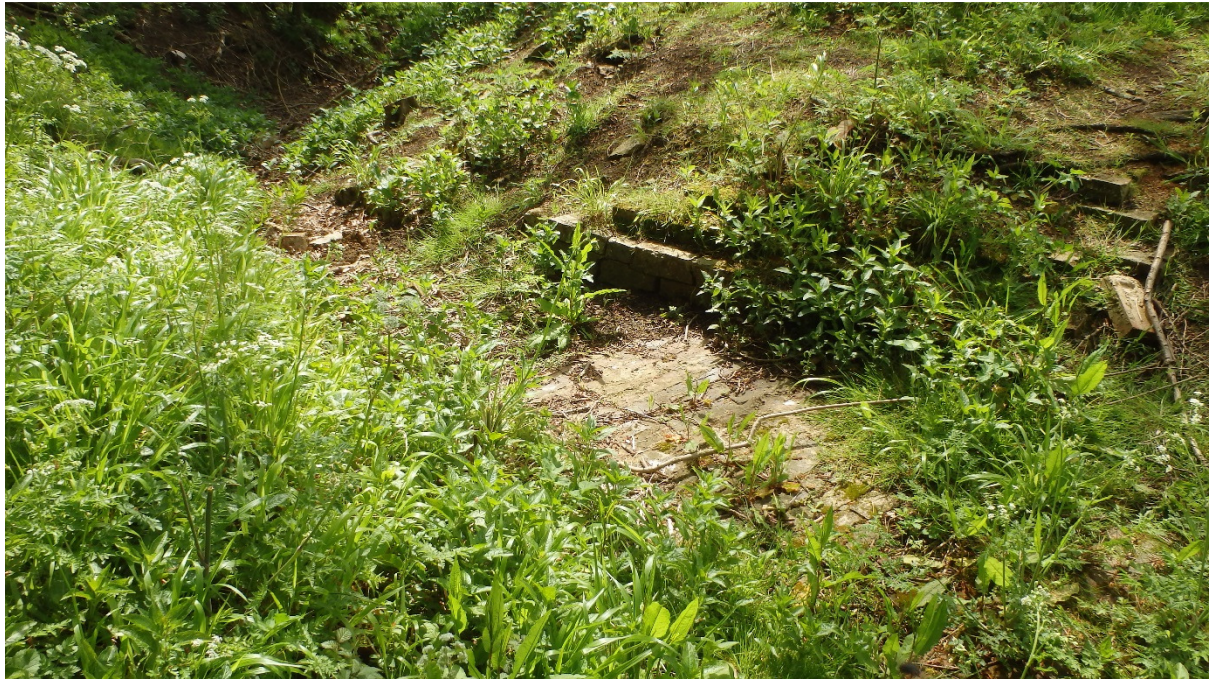
Plate 7 – Remains of spillway at north end of the dam prior to further investigation, looking southeast
