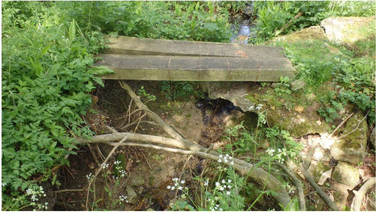
Plate 5 – Breach of dam showing former concrete repair work, looking west
