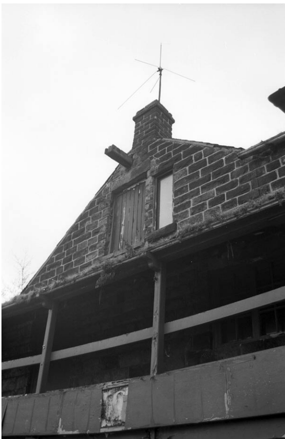
Plate 19 Eastern Gable of E-W Range, upper part showing jib over loading door, looking southwest
