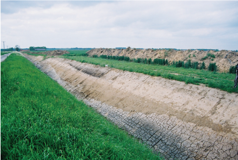
Plate 4 - View showing the profile of the Ripplingale Canal with Section 4 to left of centre, looking northwest
