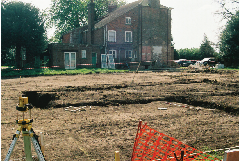
Plate 1 - View of the development area with Fishtoft Manor in the background, looking
