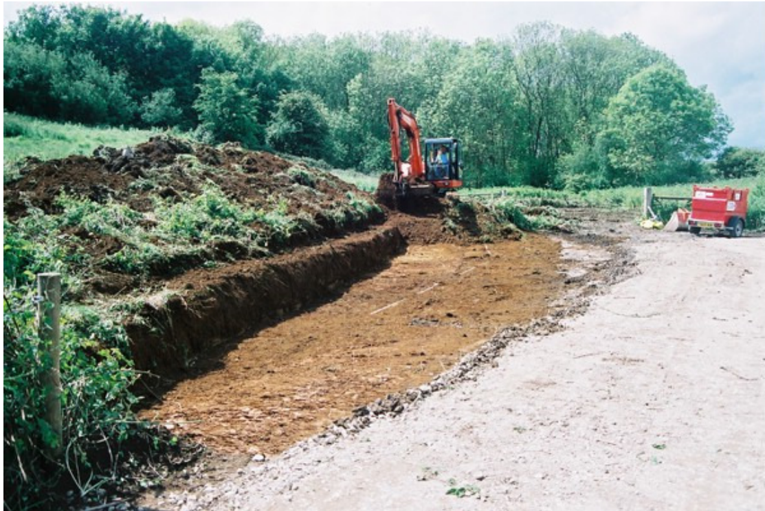
Plate 1 Southwest facing view across groundwork area, Section 1 located in left hand corner
