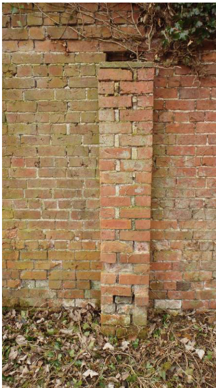
Plate 11 Brick buttress of east elevation of sawpit with stone capping and aperture above
