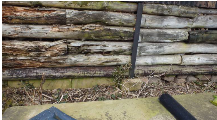
Plate 35 Detail of south elevation of Dutch barn showing iron frame on concrete pad and timber walling
