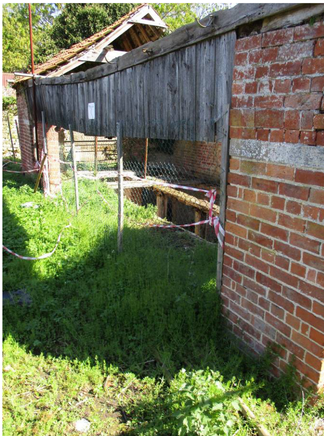
Plate 16 West elevation of sawpit showing weatherboard, opening beneath and masonry course in brickwork
