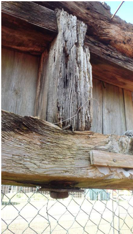
Plate 21 Detail of west wall of sawpit showing iron pin through strut joining horizontal beams
