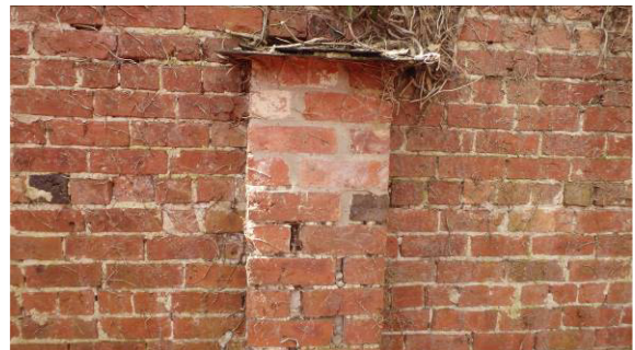
Plate 12 Repaired buttress of east elevation of sawpit, with fresh mortar and slate capping
