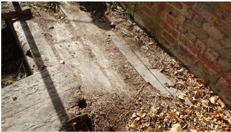
Plate 26 Detail of timber planks, joists and wood flooring at northwest of building
