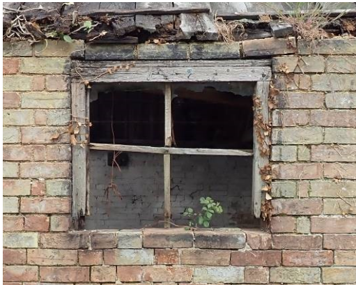
Plate 17 (above). The original window in the southeast elevation of the cattle shed surrounded by queen closers
